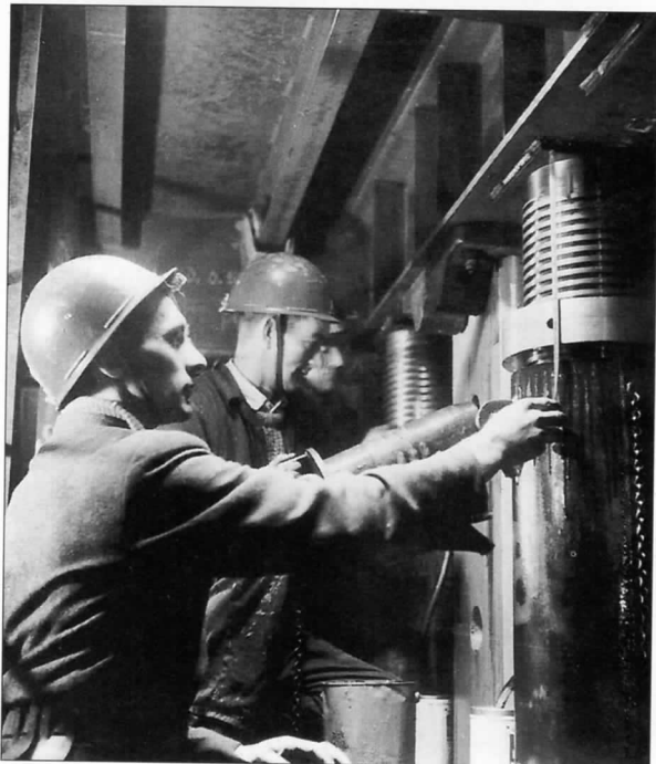
1.45 The Forth Road Bridge as built: North Tower, raising climbing structure: view of jacking corner, October 1960.
