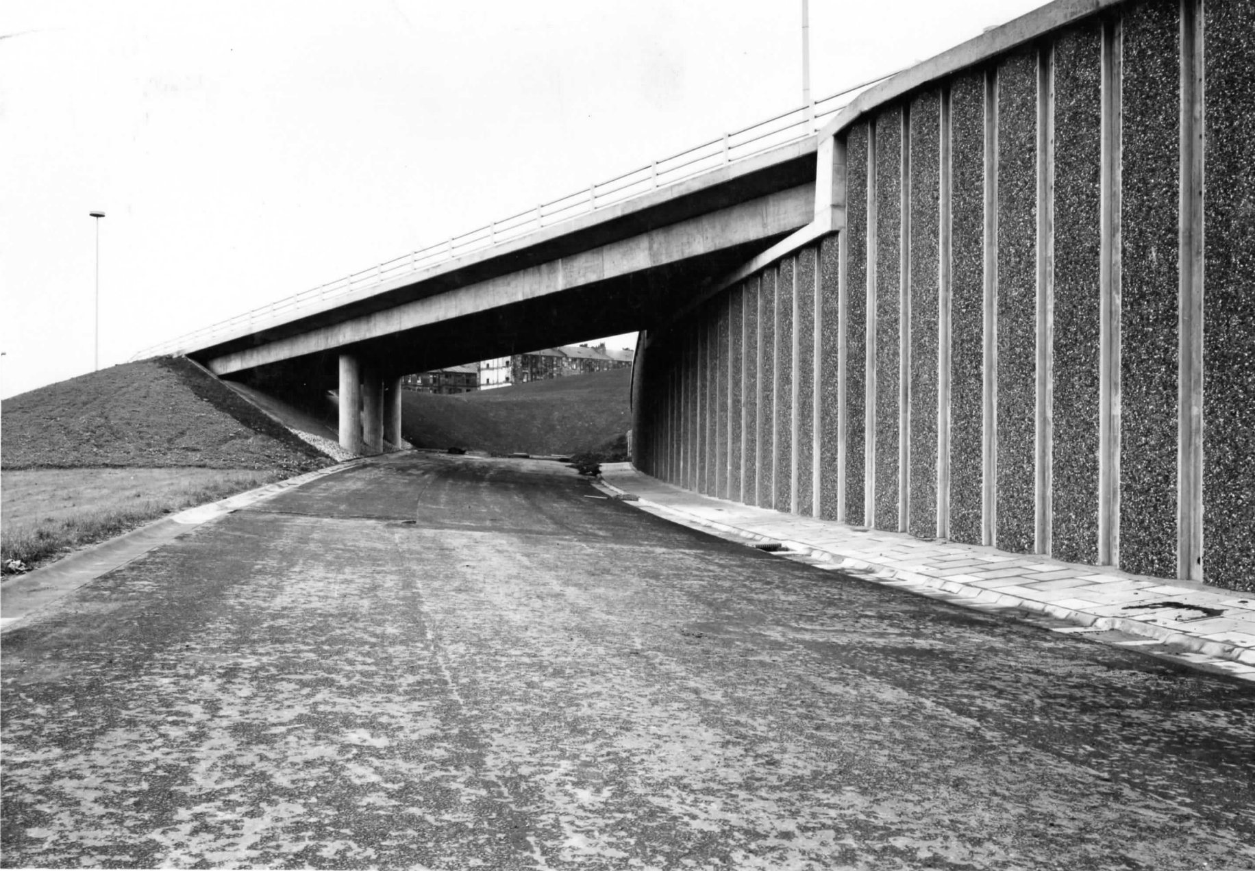
CORPORATION OF GLASGOW - WOODSIDE CONTRACT 2 Bridge 9 after finish and completion of topsoiling.
