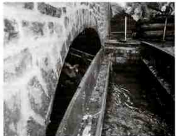
Braid Burn Bridge – 18ft span iron beams 'as found' © The City of Edinburgh Council
