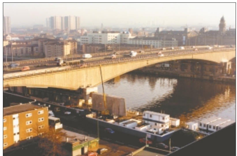
Fig 7. Existing pier slid out from below bridge
